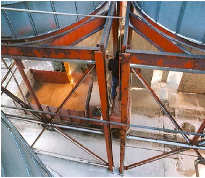
Grain dealers use overhead loadout bins to load trucks for grain transport.
